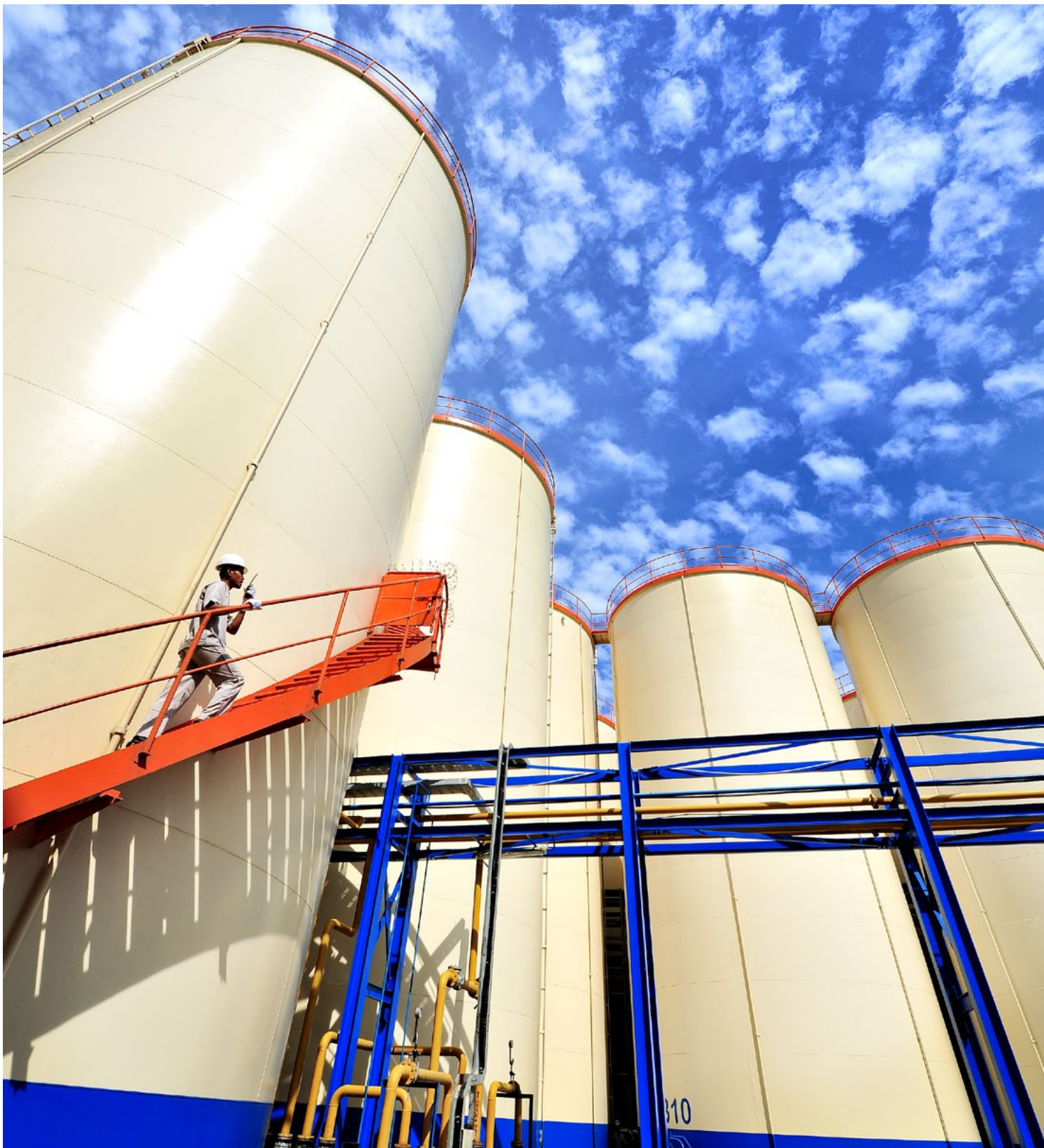
Storage tanks at Tanjung Priok refinery Tangki penyimpanan di fasilitas penyulingan Tanjung Priok
